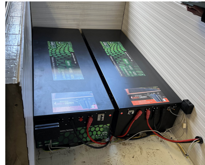
The Neilsons use 50kW batteries to store charge for overnight use.
